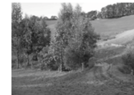
Installation of a culvert, fencing and revegetation to prevent cattle access to a stream in the Ruby Creek water supply catchment.
